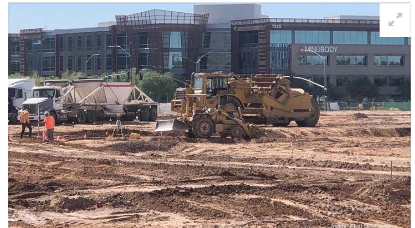
Final grading has begun at Papago Plaza for utility installation at the south Scottsdale redevelopment project.
